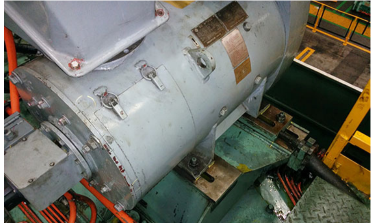
The obsolete DC motor was loud, inefficient, and required increasingly frequent maintenance in order to continue running to standards.
